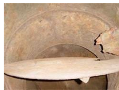
Fire damper is rusty, stuck almost open and unable to move.
