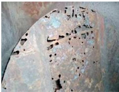
Holes in fire damper
