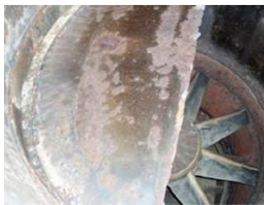
Fire damper stuck in closed position and it has been cut in half to let air escape.
